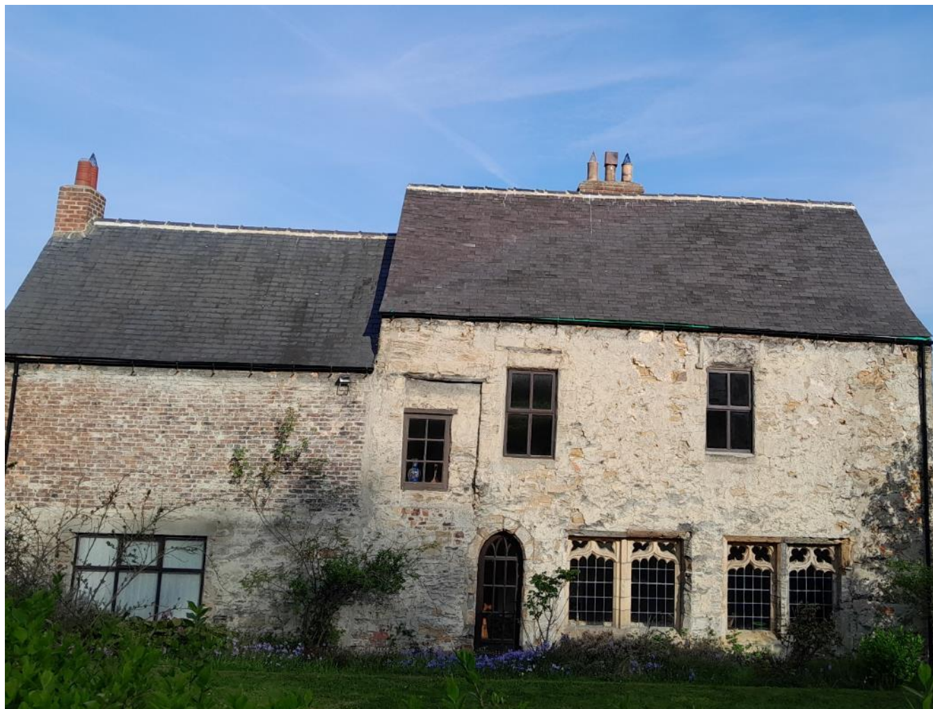
Fig 79 below. The rear of the farmhouse is particularly notable being of a rubble construction with partial boulder plinth, and including an ogee-headed entrance door, windows with Perpendicular tracery and irregular windows including a blocked opening.
