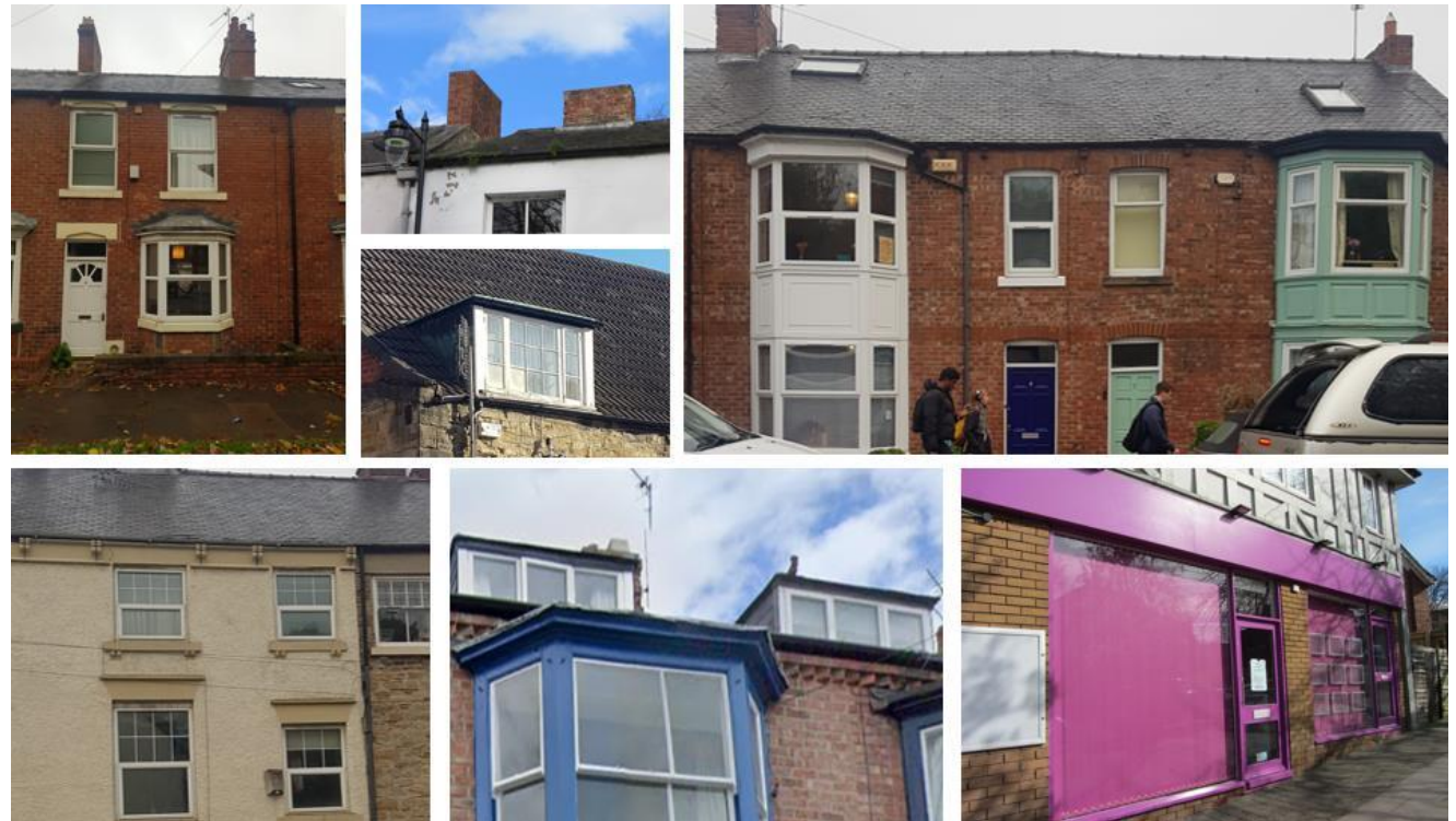
Fig 50 below. A selection of images showing examples of negative alterations, uPVC windows and doors, partly demolished chimney stacks, flat roofed dormers, a modern shop front in garish colours.
