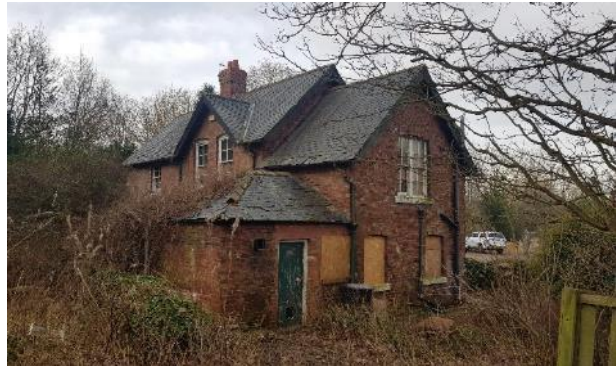
Fig 74 below. Images of the long term vacant and deteriorated group of Edwardian farm buildings at Mountjoy and the public toilets at the riverside.
