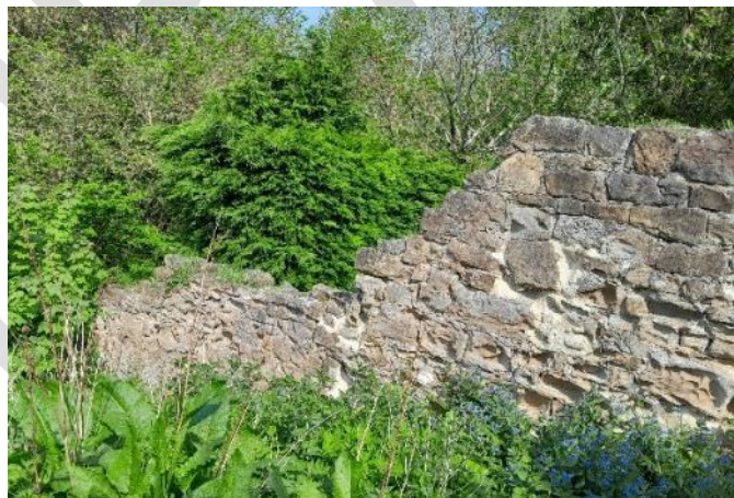
Fig 30 below and right. A selection of images showing different parts of the stone garden walls and the various condition issues.
