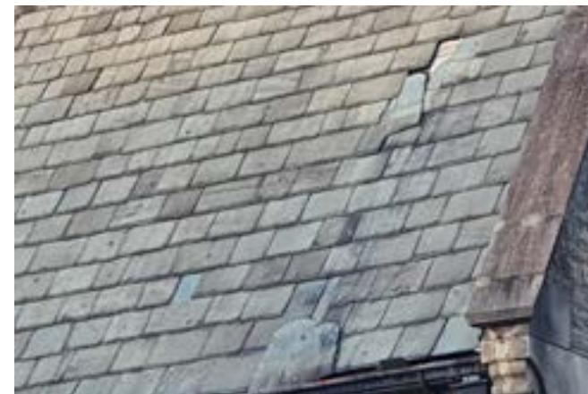
Slipped slates can quickly lead to internal damage
