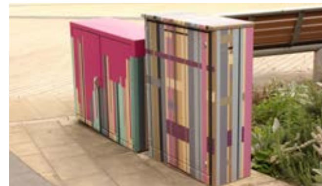
Consider combining artwork with street furniture such as telecoms and traffic cabinets as in this example in Barnsley which adopts colours which effectively 'camouflages' the cabinets
