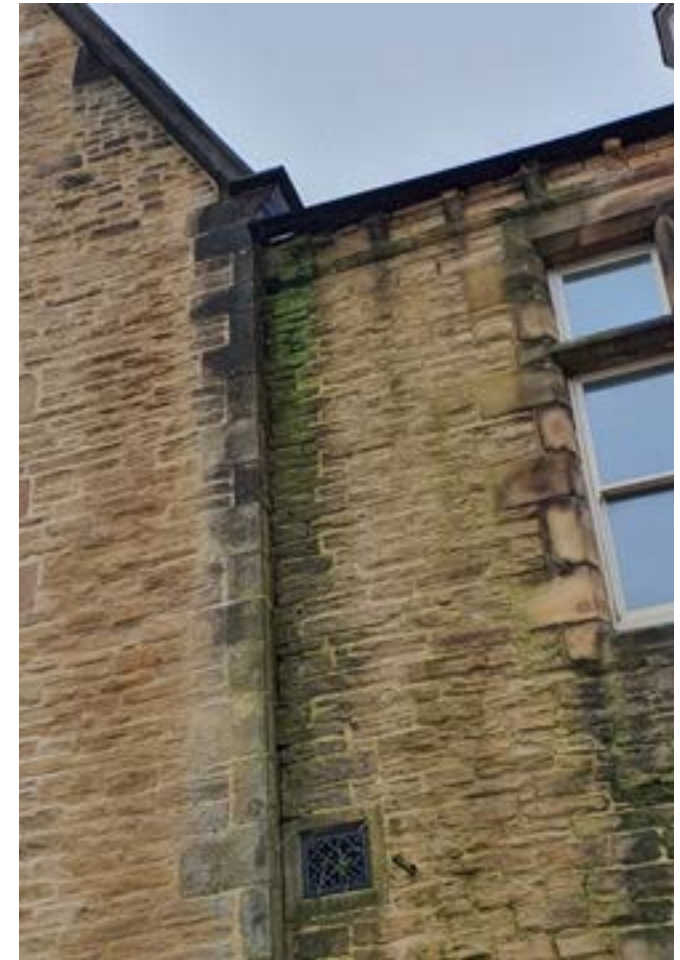
Poor maintenance such as blocked or missing gutters can quickly lead to issues
