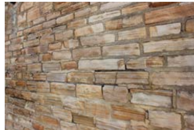
Poorly pointed stone wall
