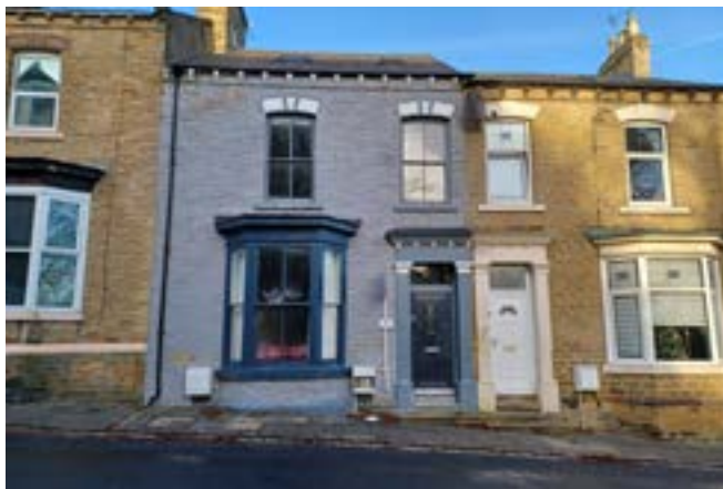
Painted stonework is both damaging to the building’s fabric but also disrupts the appearance of an otherwise uniform terrace
