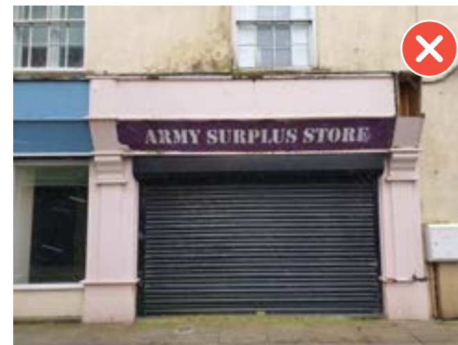
Solid roller shutters create an inactive and unpleasant streetscene when closed
